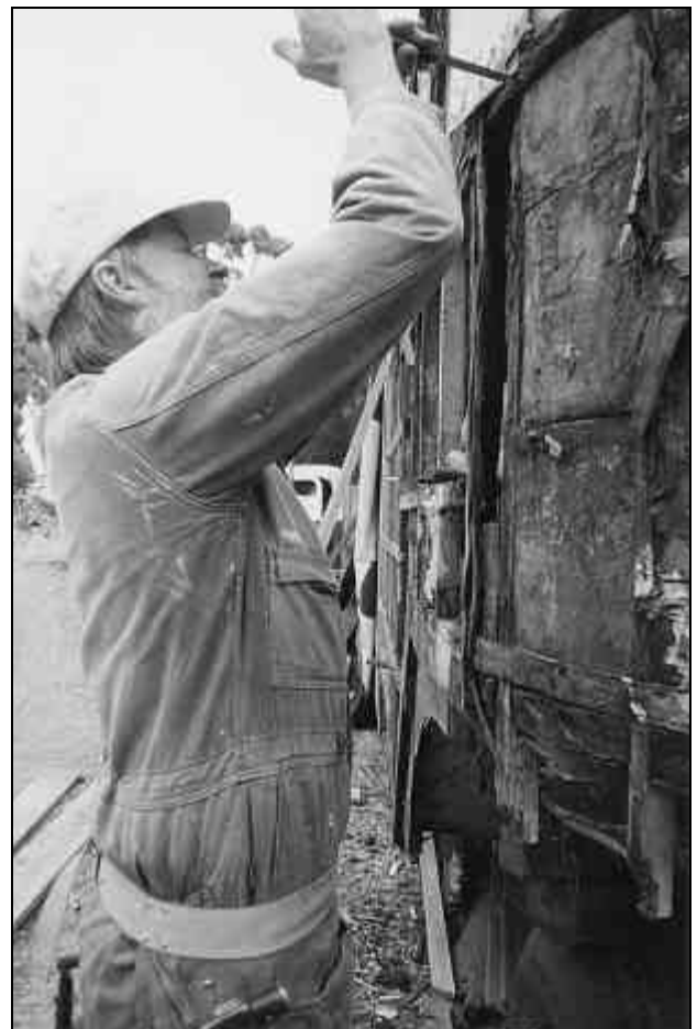
The boys had reached the stage of pulling the aluminium cladding off the front curved part of the van, and Graham armed with a handsaw was cutting out the blocks of insulation. Action photos were taken (see above).
