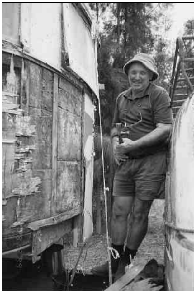
Dick is about to attack the aluminium cladding which had to come off the front corner
