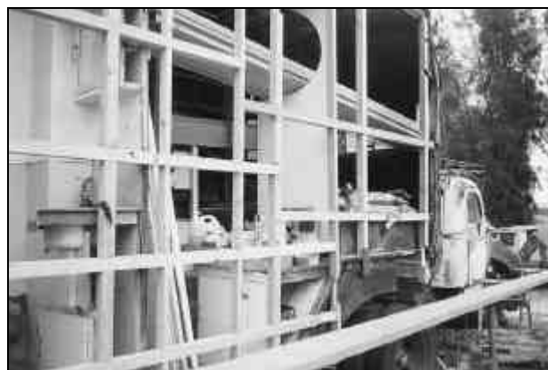
Some of the new framing viewed from the rear quarter - the plank is for standing on!
