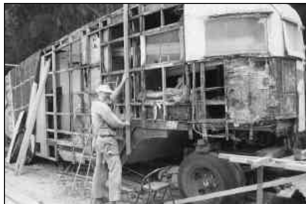
Graham measures up one of the replacement vertical battens - the size of only one side of the monster would deter any sane mortal!
